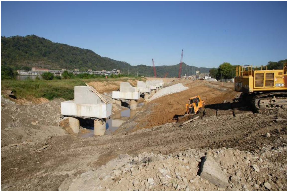
Figure 1.2 Marmet Lock Upper Guide Wall Intermediate Piers during construction (courtesy of Huntington District)
