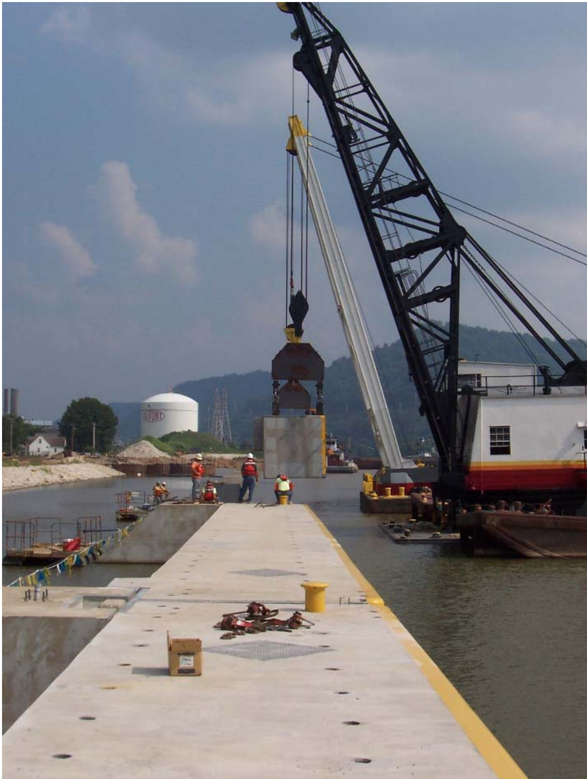
Figure 1.4 Lifting and setting the Marmet approach wall beams (courtesy of Huntington District)
