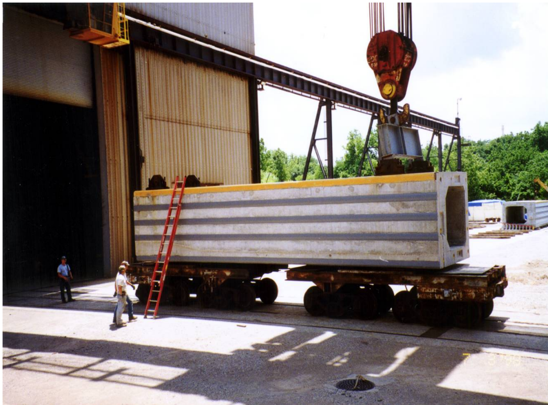
Figure 1.9 Side view of one of three match-cast guide wall box beams at the fabrication yard (courtesy of Huntington District)
