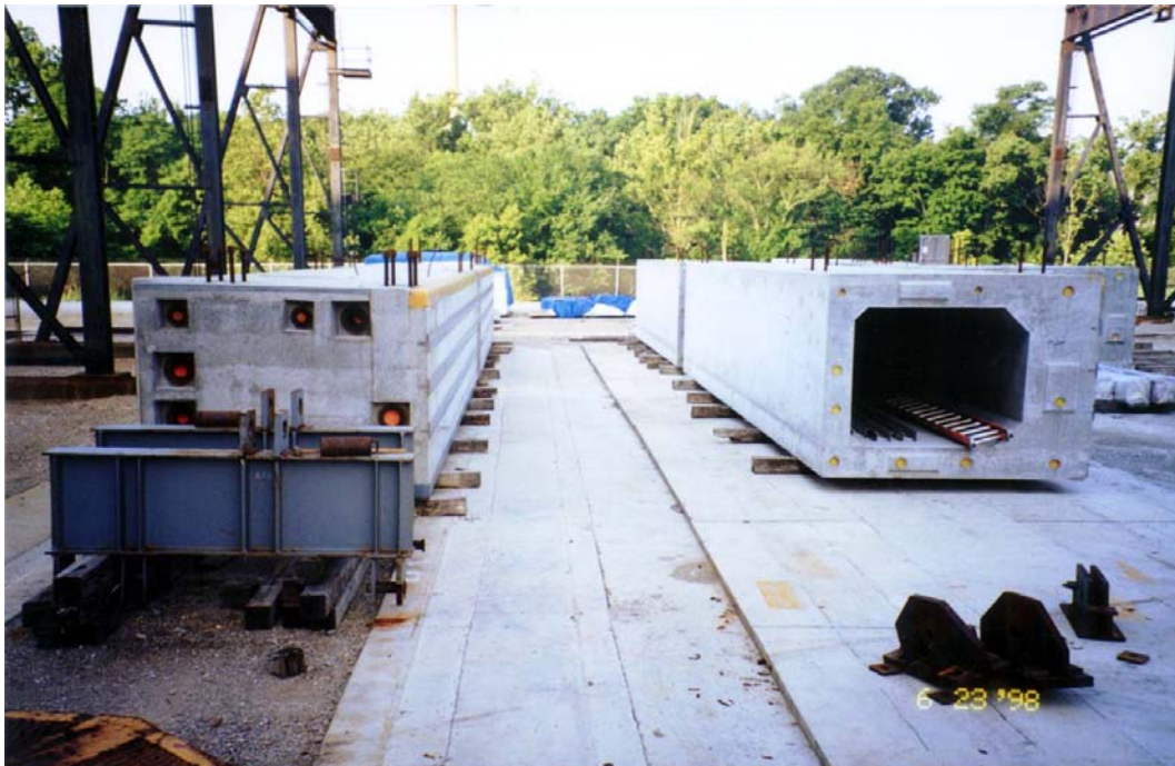
Figure 1.8 End view of the match-cast guide wall box beams at the fabrication yard (courtesy of Huntington District)
