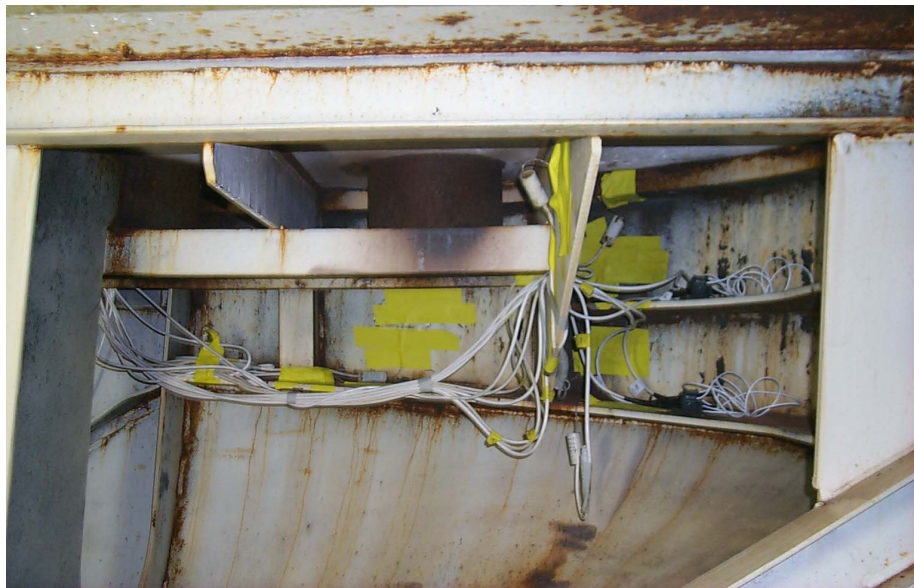
Figure 5.8. Layout of strain gages under deck for baseline experiments (Note: Yellow tape covers the strain gage locations)
