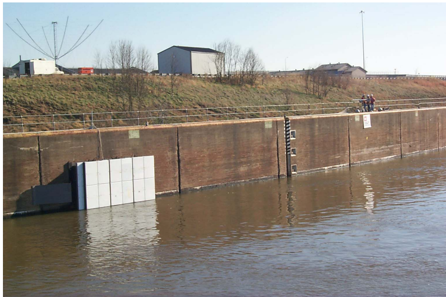
Figure 5.2. Locations of impact zones on upper guide wall at Gallipolis Lock (Note: Fenders are on left; concrete impacts are on right below white sign)
