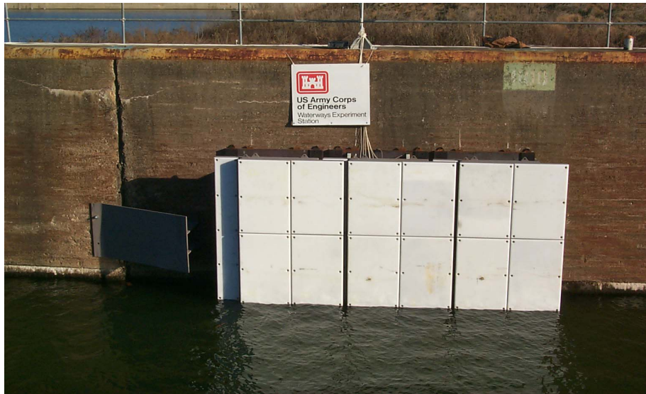
Figure 6.1. As-built prototype fendering system on upper guide wall at Gallipolis Lock and Dam
