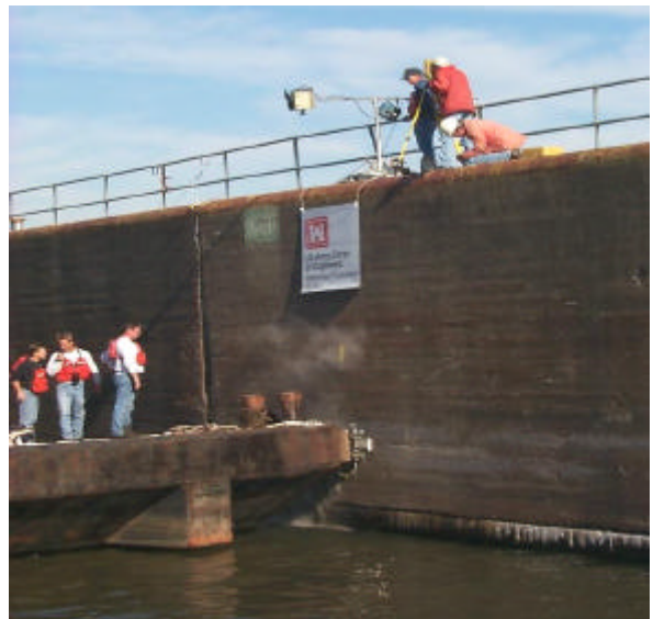
Figure 1.3. Barge impacting on lock wall without armor (note concrete dust)
