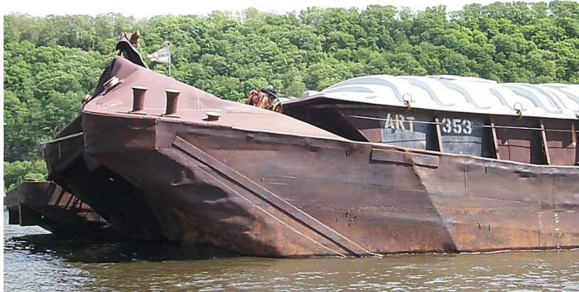
Figure 1.2. Barge damage caused by high energy impact with a bullnose structure (Photo credit: U.S. Army Corps of Engineers)
