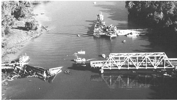
Figure 2.2 Failure of the Big Bayou Canot railroad bridge in Alabama (1993) after being struck by a barge flotilla
