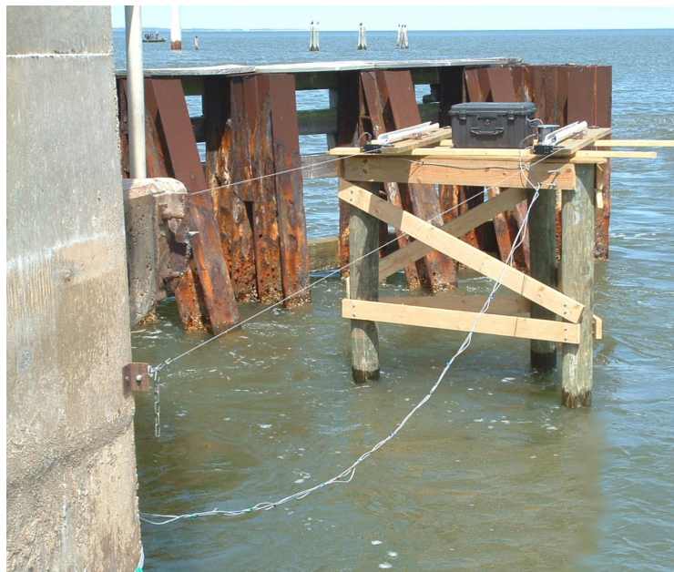
Figure 6.31 Stationary timber platform on east side of Pier-1 as viewed from a position adjacent to the pier
