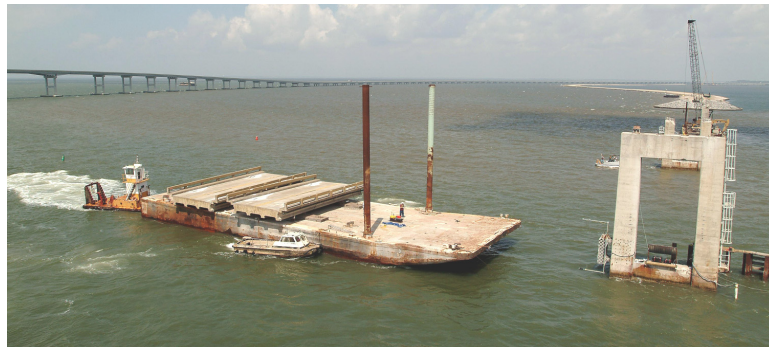
a) Test barge with payload consisting of two 55 ft. long bridge spans
