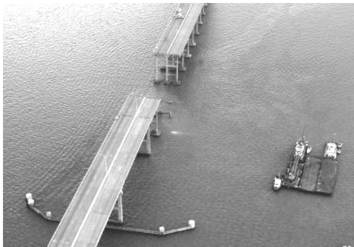
Figure 2.3 Collapse of the Queen Isabella Causeway Bridge in Texas (2001) after being struck by a barge flotilla
